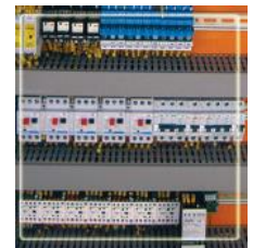
Electrical components from well-known European manufacturers are easily available
